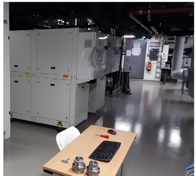
Figure 2. A view of the energy central, seen from the middle of the room. The rather sparsely equipped “work station” hints at the level of automation – necessary human intervention is reduced to a minimum.
